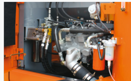
Grouped remote filters and inspection points
