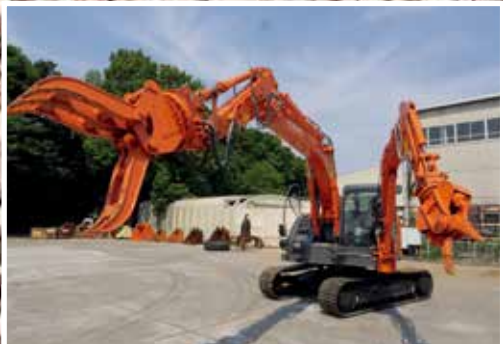
ASTACO (Advanced System with Twin Arm for Complex Operation)
