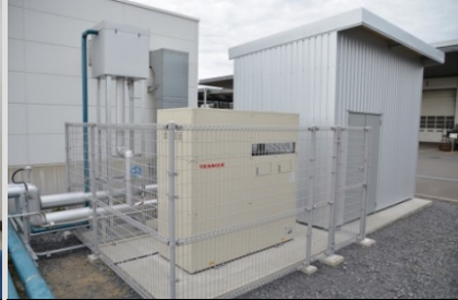
Cogeneration systems* (Hitachinaka Works)
