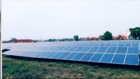
Solar panels (India Works)
