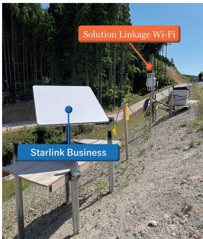
Solution Linkage Wi-Fi(親機)とStarlink Businessの接続
